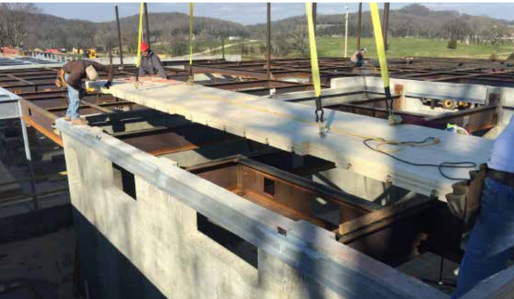
Left: In 2014, TSE was an early adopter of CLT gravity systems on this mixed-material residence.
